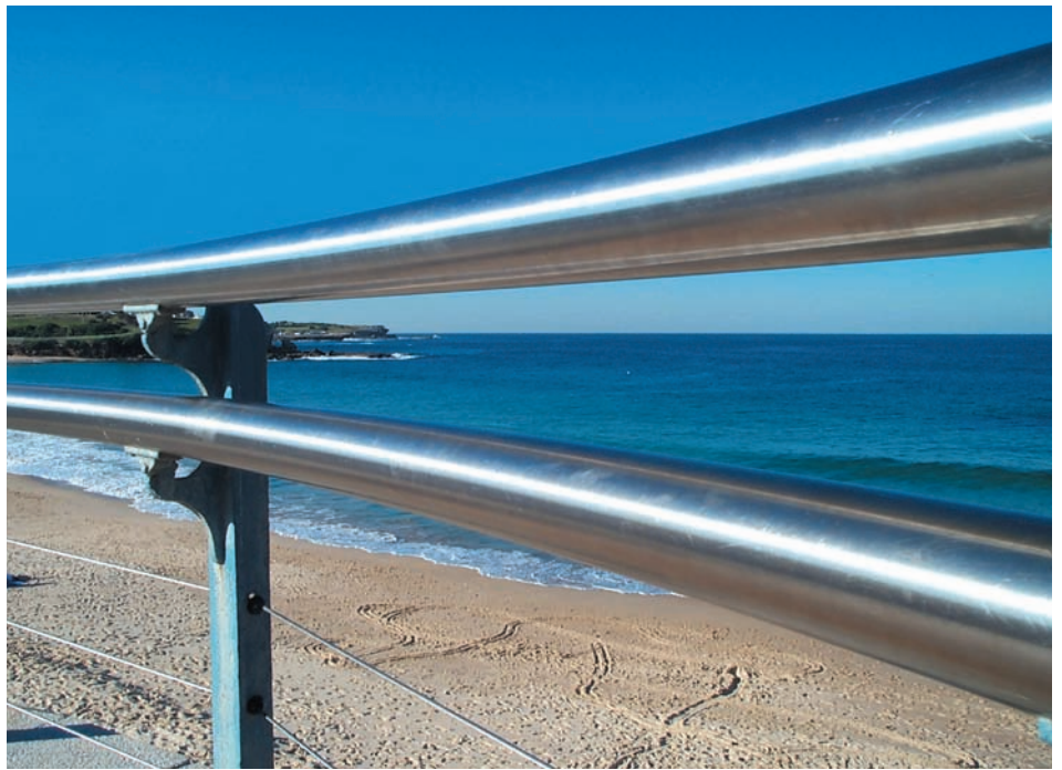
Successful use of stainless steel after more than 14 years service in a coastal environment.
